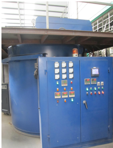
Steam treatment furnace(2 pcs)
